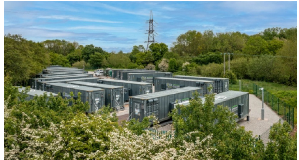
Fideoak battery site near Taunton (28 MW)
